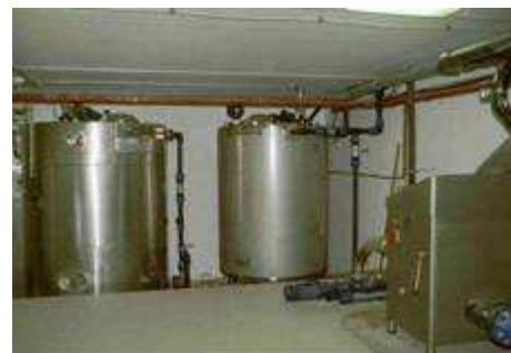
Fig. 9: Mixing and hygienisation unit, (source: Otterwasser)
